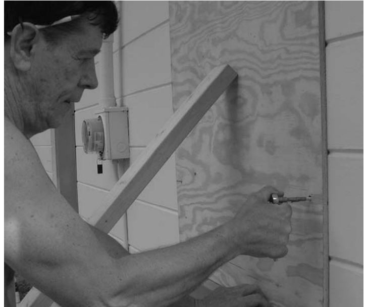
Tom uses a 1/4" ratchet and an adapter that comes with the fastener kit to install the studs into the masonry. Below is the plywood with the wing nut install and ready for the wind.
